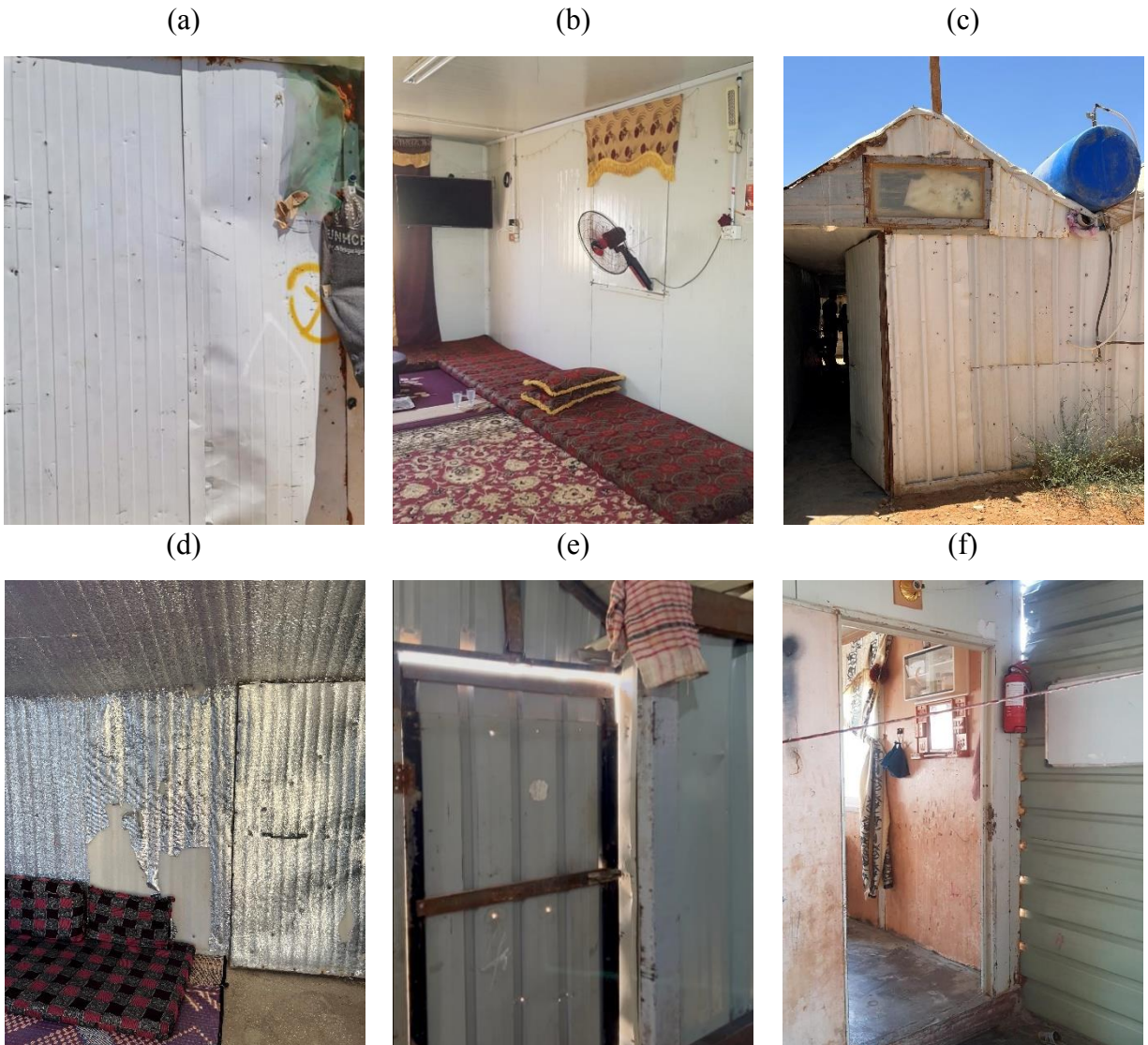
448 Figure 3: Examples of cases where walls and roofs have holes and gaps: a) An external wall with holes- Zaatari 449 camp- Shelter 7 (Alshawawreh, 2021), b) An indoor wall with slots from relocating the window- Zaatari camp- 450 Shelter 3 (Alshawawreh, 2021), c) An external wall with holes and slots- Azraq camp- Shelter 3 (Alshawawreh, 451 2022), d) An indoor lining with a ripped-off aluminium foil layer- Azraq camp- Shelter 1 (Alshawawreh, 2022), e) 452 Door with holes and air gaps around- Azraq camp- Shelter 1 (Alshawawreh, 2022), f) Air gaps in the connection 453 between the self-built wall and the provided shelter- Zaatari Camp- Shelter 3 (Alshawawreh, 2021).
