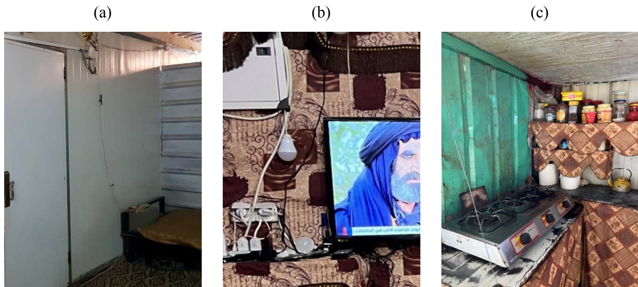
387 Figure 1: Examples of possible causes of fire ignition: a) Unsafe electric cords- Zaatari camp- Shelter 2 388 (Alshawawreh, 2021), b) Overloaded circuit close to fabric lining- Azraq camp- Shelter 3 (Alshawawreh, 2022), c) 389 Open flame close to fabric lining in a kitchen- Azraq camp- Shelter 2 (Alshawawreh, 2022)
