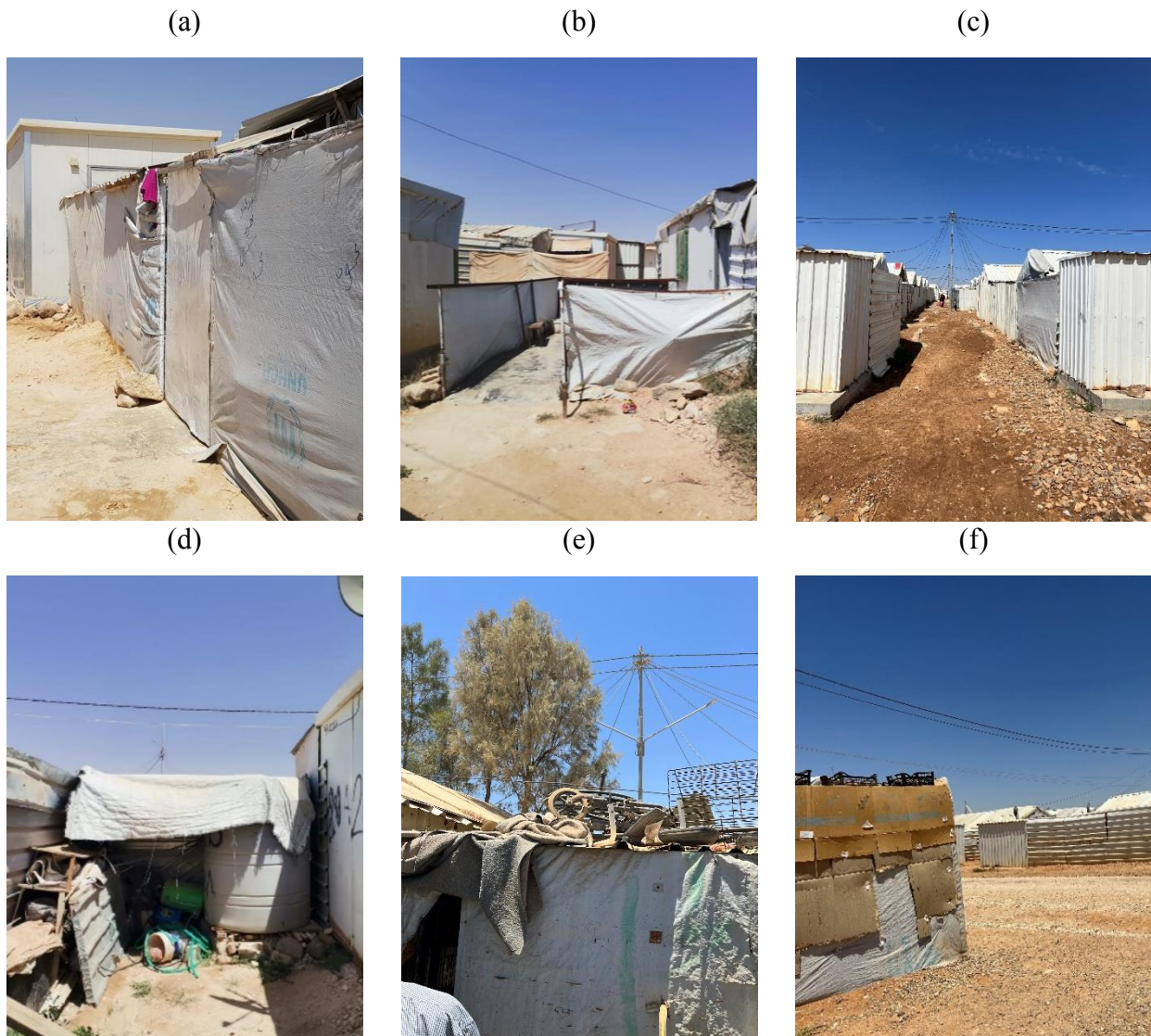
518 Figure 6: Exterior photos in the camps that show how fire could spread between different structures: a) Self-built 519 extensions- Zaatari camp- Shelter 5 (Alshawawreh, 2021), b) Narrow pathway between shelters- Zaatari camp- 520 Shelter 6 (Alshawawreh, 2021), c) Rows of shelters- Azraq camp- Street view (Alshawawreh, 2023), d) Outdoor 521 stored materials- Zaatari camp- Shelter 7 (Alshawawreh, 2021), e) Over-roof materials- Azraq camp- Shelter 2 522 (Alshawawreh, 2022), f) Over-roof materials- Azraq camp- Street view (Alshawawreh, 2022).
