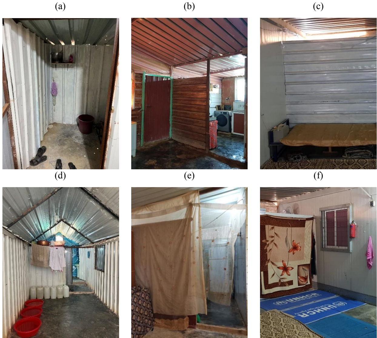
493 Figure 5: Interior photos of some shelters where additions could accelerate the fire spread within the shelter: a) Self- 494 built toilet- Azraq camp- shelter 3 (Alshawawreh, 2022), b) Self-built kitchen- Zaatari camp- shelter 4 495 (Alshawawreh, 2021), c) Self-built partition dividing a shelter- Zaatari camp- shelter 5 (Alshawawreh, 2021), d) 496 Self-built hall and toilet- Azraq camp- shelter 1 (Alshawawreh, 2022), e) Self-built short wall enclosing a toilet- 497 Zaatari camp- shelter 7 (Alshawawreh, 2021), f) Self-built short partition enclosing a storage- Zaatari camp- shelter 498 5 (Alshawawreh, 2021).
