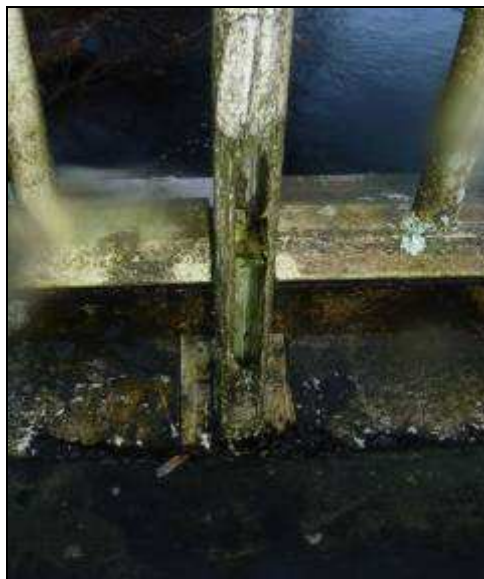
Figure 17. Impact damage to the bottom of a parapet post (December 2011).
