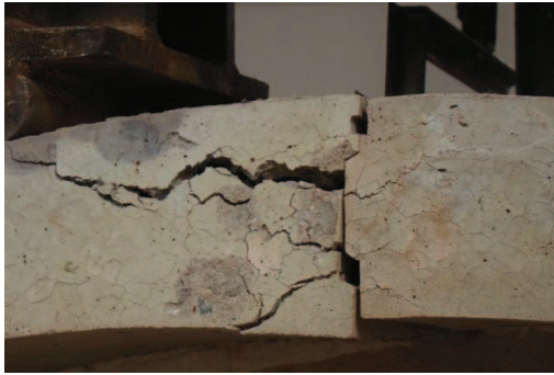
(a) Joint concrete failure (RCJ5)
