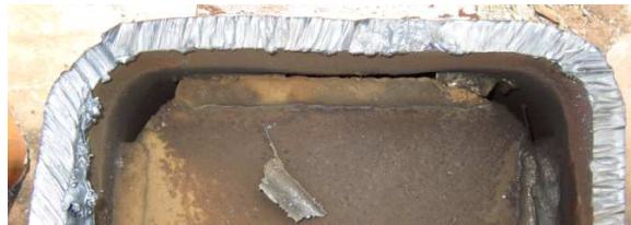
Fig. 9. Separation between the bottom inner-diaphragm and column wall on the west side in Specimen SI-WB-2.
