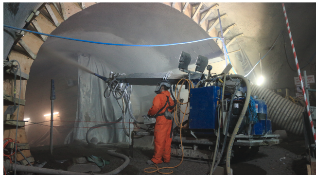
Fig. 1. Concrete spraying in a freshly excavated tunnel, using a 5-DoF concrete spraying unit. A skilled operator controls the device on a per-actuator level via a number of joysticks. Image courtesy of Costain Laing O’Rourke Joint Venture.
