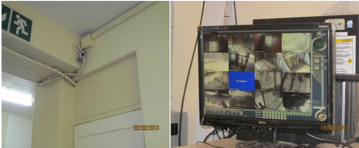
Image 3: CCTV surveillance equipment inside social housing buildings, Hillbrow (photographs by the author)
