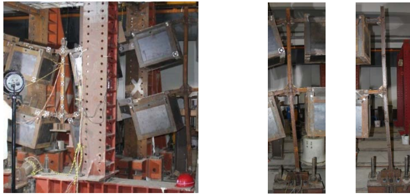
Fig. 3 Global damage of FRAME2 (middle and right photos show damages of columns)
