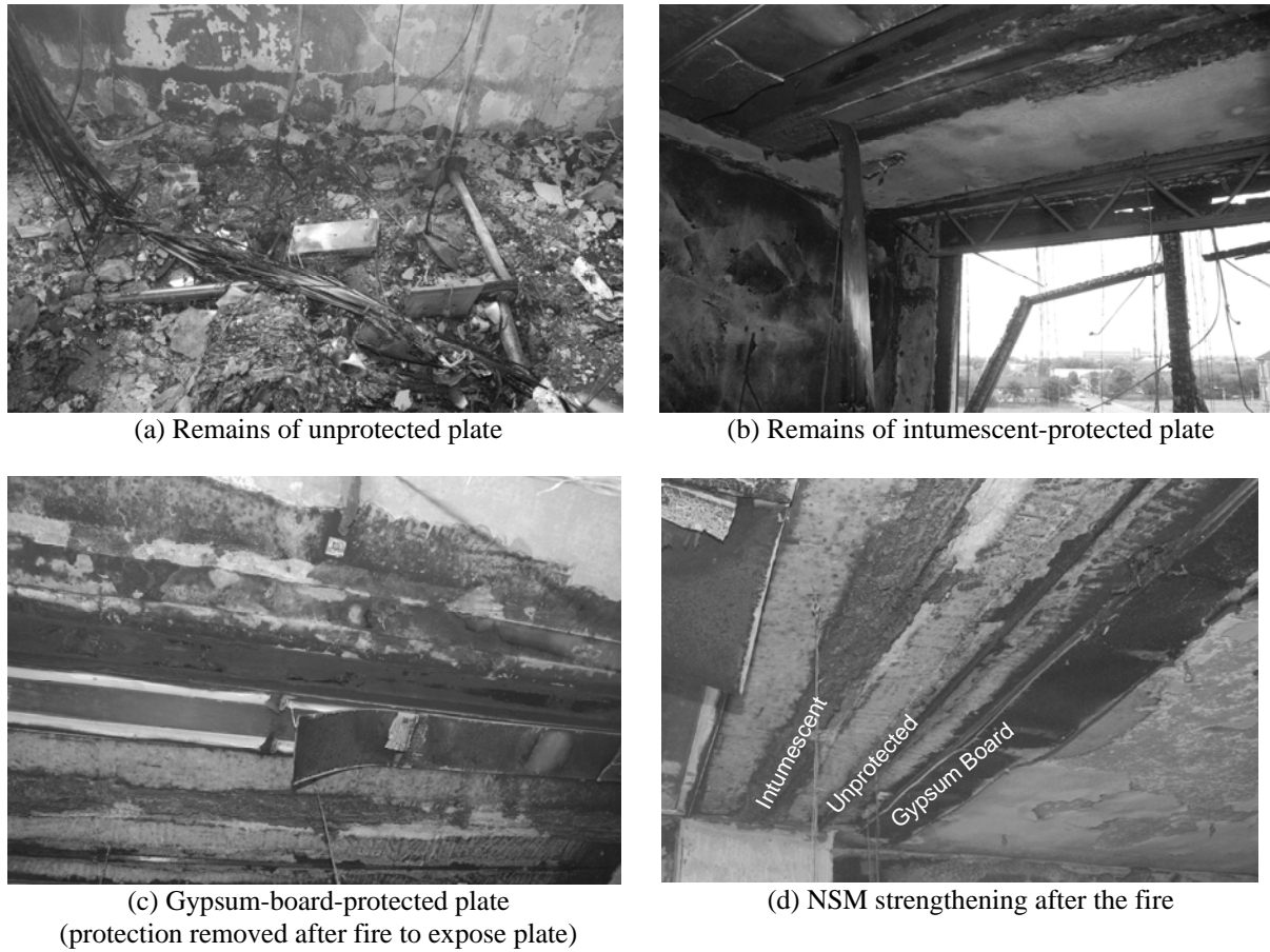
Figure 3. The condition of the bonded strengthening after the fire.
