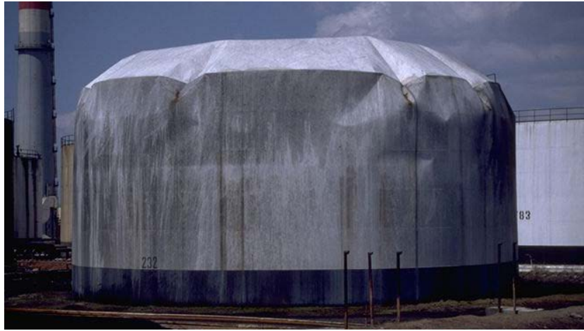
Figure 2: Tank roof damage due to sloshing [6].
