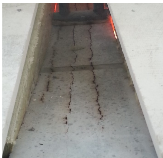
470 471 Figure 20 – Longitudinal splitting cracks at the unexposed surface of Slab #4 shortly before failure.
