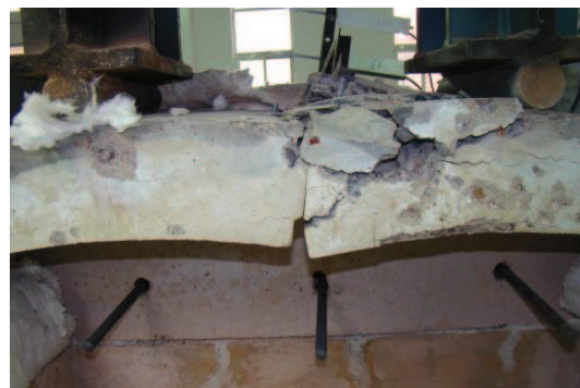
(g) Joint concrete failure (RCJ4)
