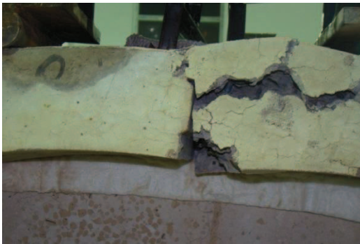
(c) Joint concrete failure (RCJ6)
