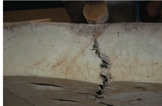
(h) Concrete fracture (HFRCJ4)
