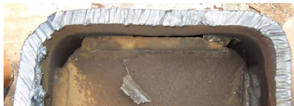
Fig. 9. Separation between the bottom inner-diaphragm and column wall on the west side in Specimen SI-WB-2.
