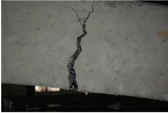
(a) Steel fiber failure under mechanical loading
