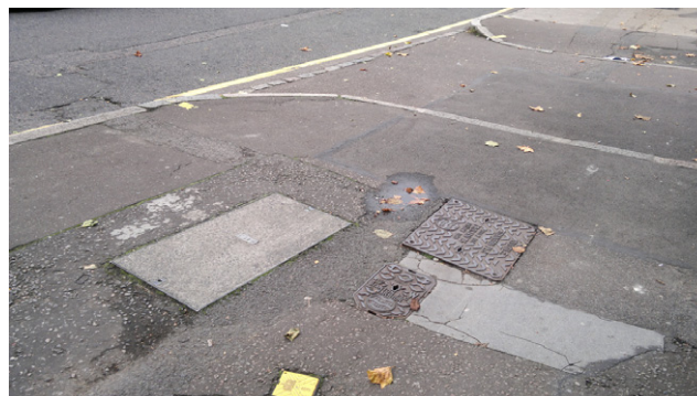
Figure 3. Changes in levels due to manhole covers
