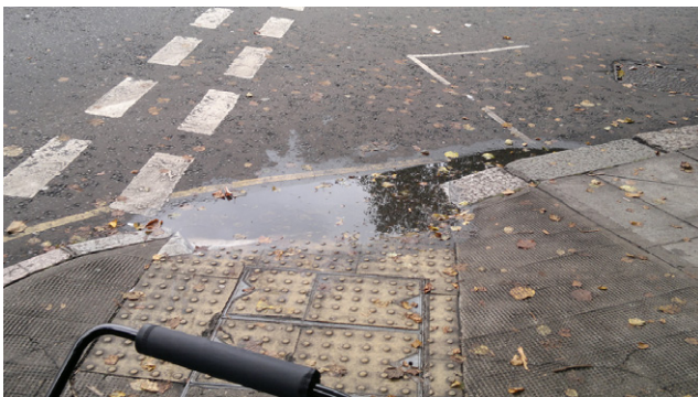
Figure 14. Uneven pavement and accumulation of water makes this road crossing challenging
