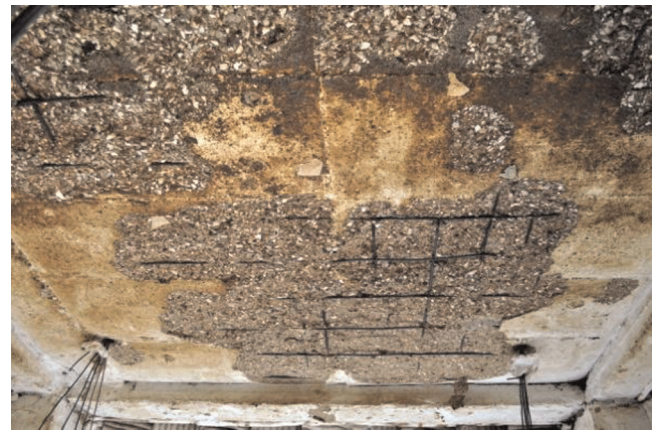
Fig. 12. Spalling in roof slab after fire.
