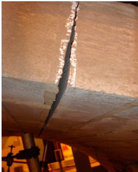
(a) Intrados Crack C_{N1}
