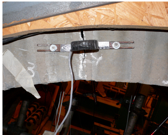
(b) Extrados Crack C_{NA}
