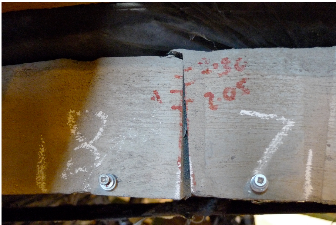
Figure 17 - Mixed-mode flexural and shear failure at intrados crack ( C_{S1} ), on the west side of the bridge
