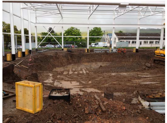
Fig. 5. Initial excavation of pit for the containment tank with the steel frame of the building erected before excavation commenced.
